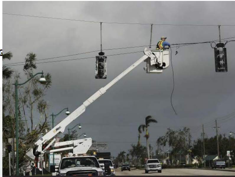
An electrical worker repairs stoplights the morning after Hurricane Irma swept through Naples, Florida.
